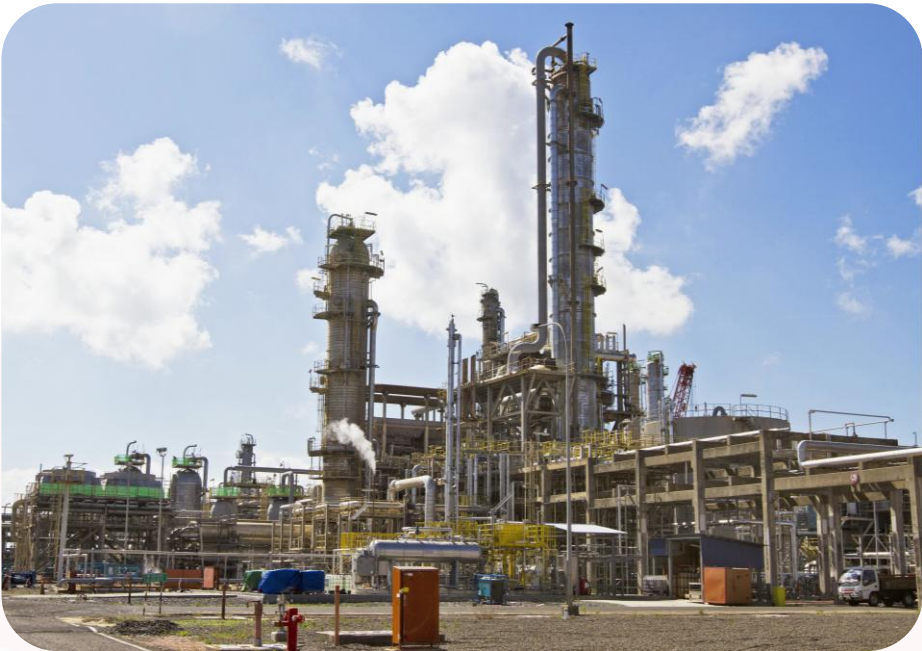
Gas Processing Plant, Kerteh
